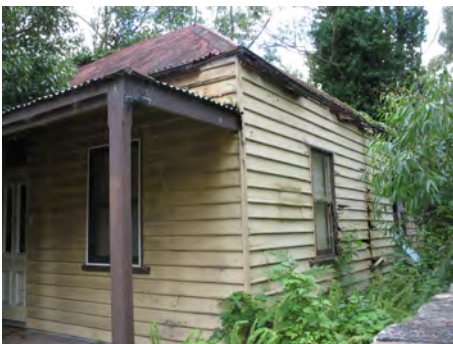
11 Mark Street – still mouldering away
